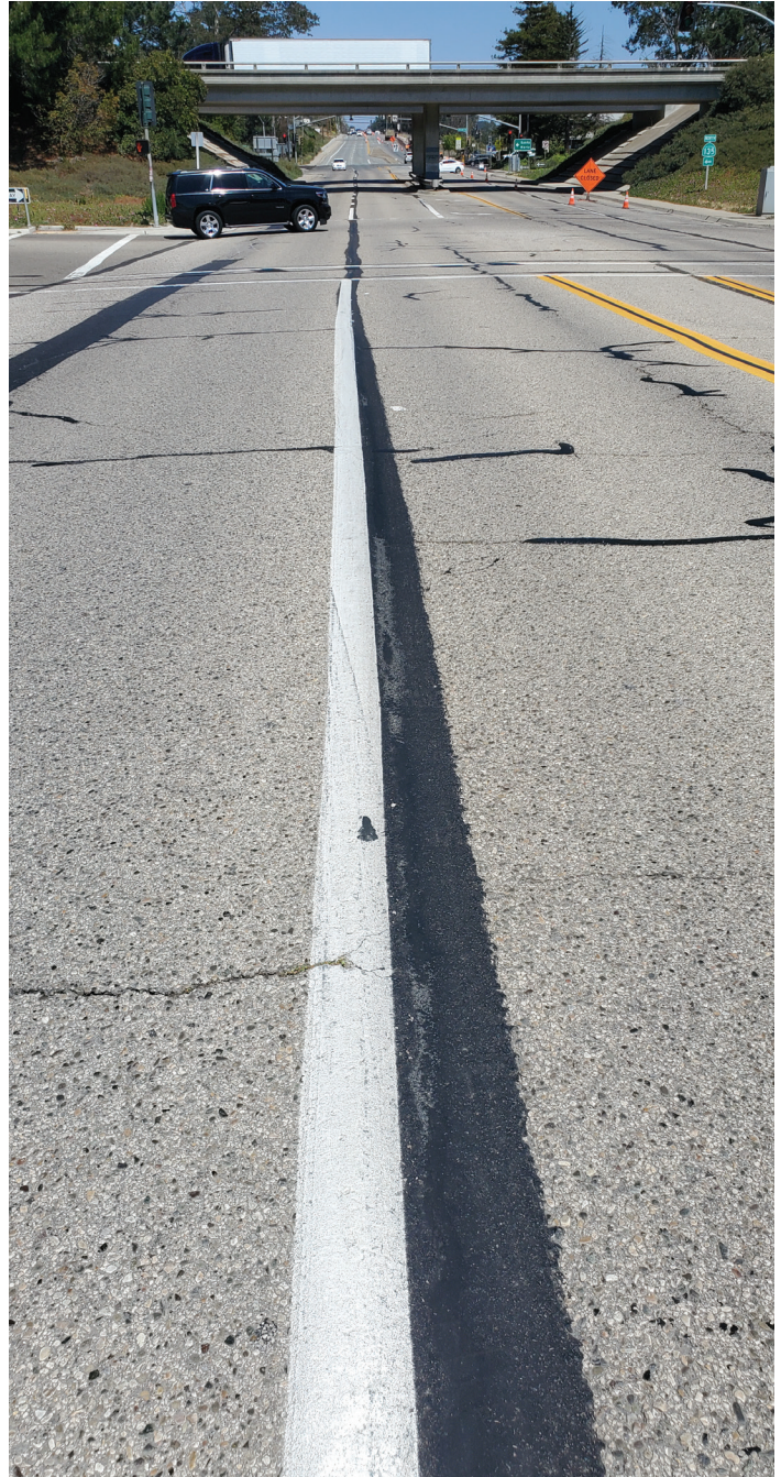
The crew applied 100 yards of the Mastic One material at a time with the drag box, saving the county countless hours.
